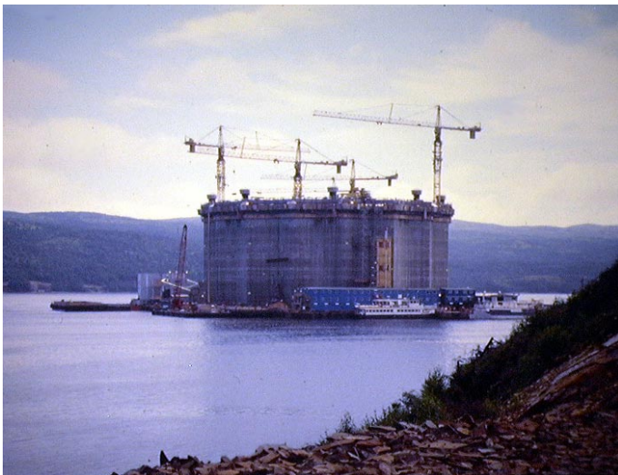
The Hibernia Project Gravity Base Structure under Construction at Bull Arm, N.L., July, 1995.
