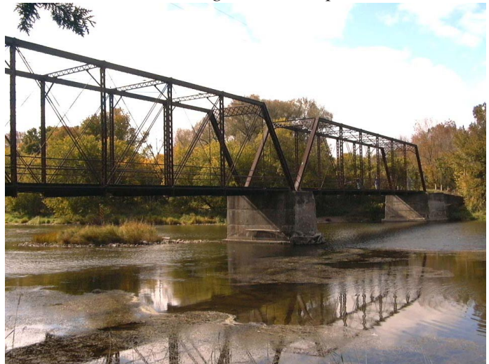
19th Century Ball's Bridge Spanning the Maitland River near Little Lakes, Ontario, October, 2004.
