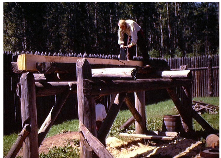
Lengths of Wood Being Sawn in the Sawpit Scaffold, Fort William, Thunder Bay, Ontario, August, 1980.
